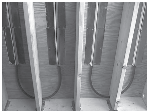
7/8" PEX in a floor Joist application
