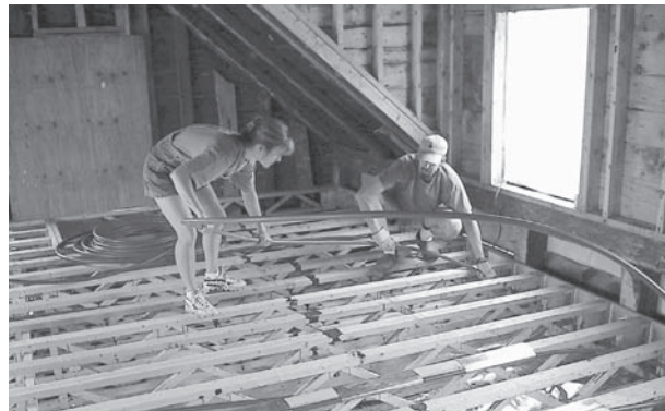
Trusses are so wide open that running 7/8" PEX through the bays becomes a very simple job.
