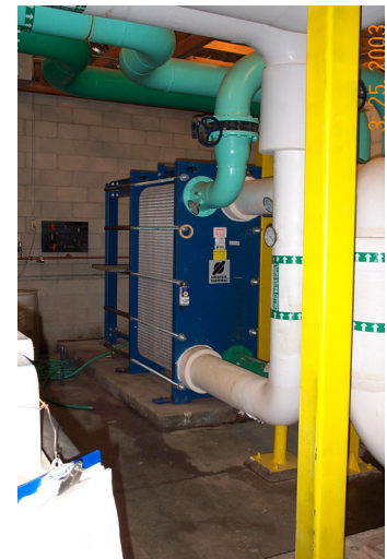
Figure 3 - This plate and frame heat exchanger may be of more value elsewhere
