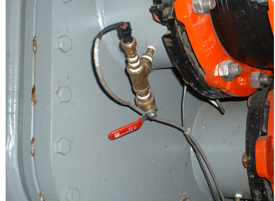
Figure 7 - Current installed condition of the temperature sensors for the chillers. The sensor head is the black portion of the assembly with the wires attached to it. The actual sensing element extends from the head into the tee towards the valve with the red handle. The temperature it is supposed to be sensing is the water inside the line above it.
