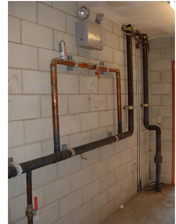
Figure 16 - Blackened domestic water piping in the Spa area
