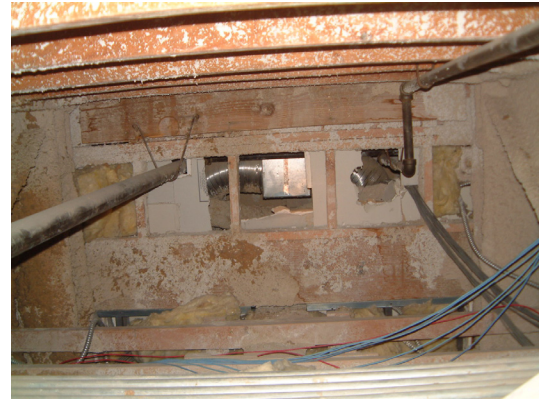
Figure 20 - Above ceiling openings between return plenum and the area served by the turbine ventilators
