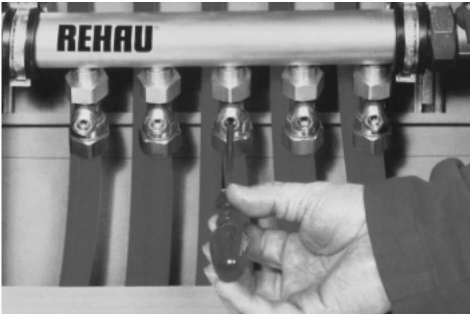
Fig. 5.25: The design will have specified how many turns each valve will require to balance each circuit.
