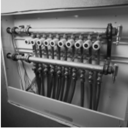
Fig. 5.17: Wall cavity manifold cabinet.
