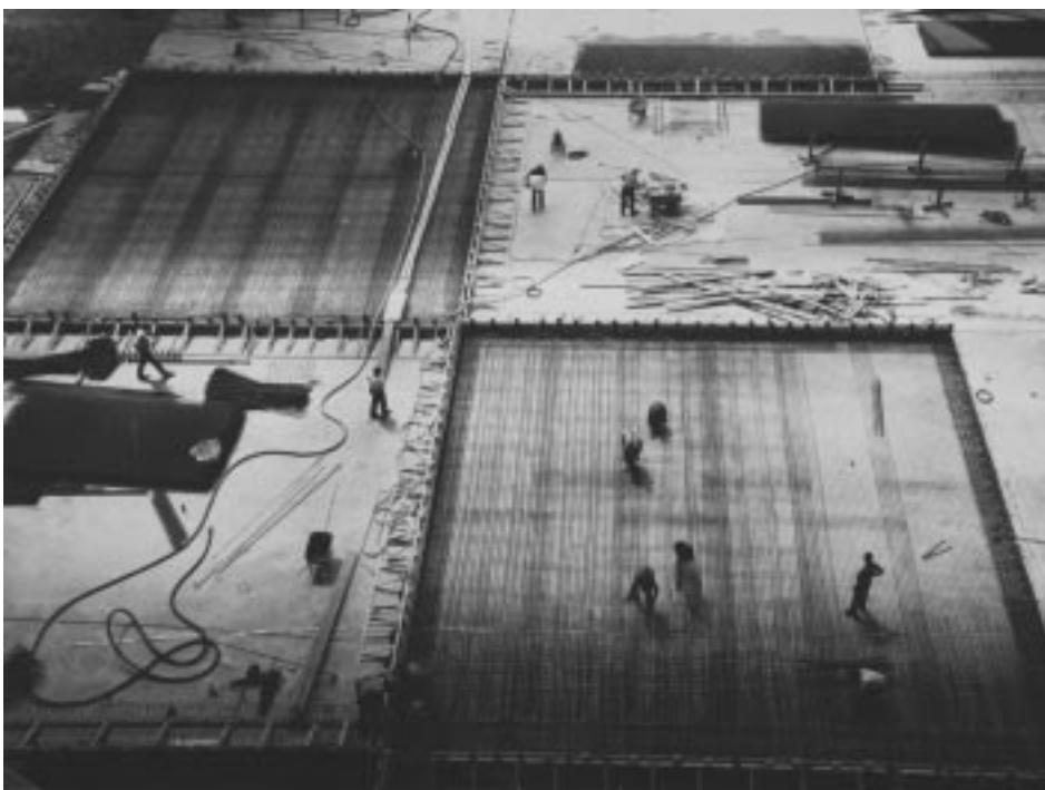
Fig. 1.2: Floor of aircraft hangar incorporating RFH system.
